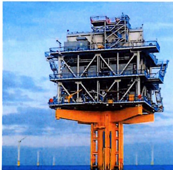
Image 4 : Typical Offshore Substation on jacket foundations
